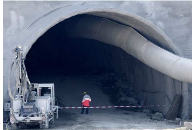
Figure 5 Exploison in Šibeník tunnel [8]
